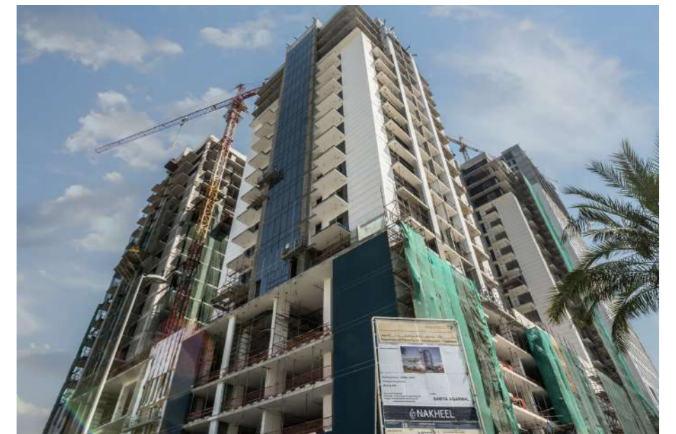
From Left - Right: On - going construction activites of Vita Grande, 7 Park Central and The East Crest as on April 2024.
