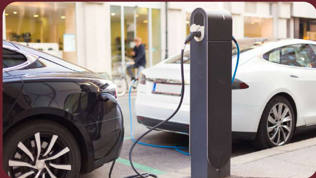
ELECTRIC CARS CHARGING STATION
