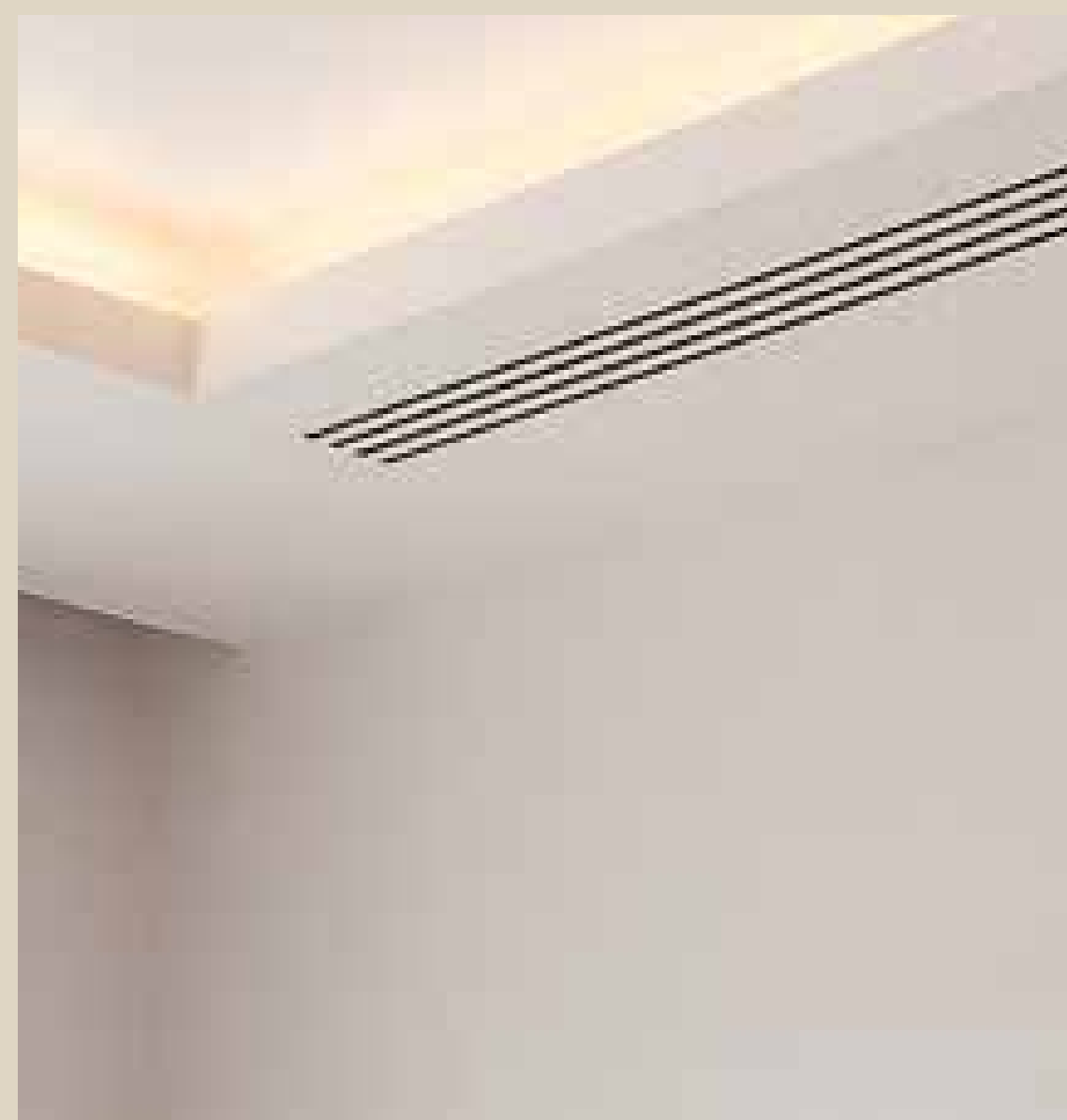
Air Condition “Ceiling-Mounted : Daikin”
